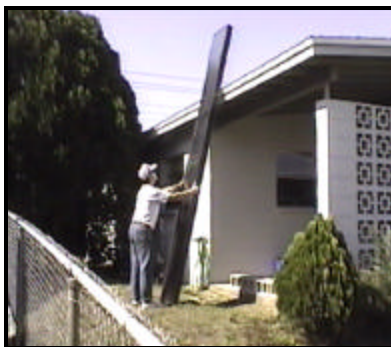
Protect Edge of Roof with a Tarp and Lean Collector Against Roof
